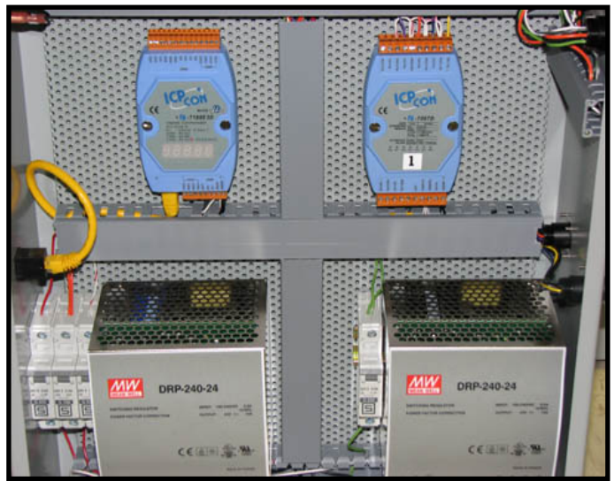
I-7188E3 and I-7067D with power supplies for remote panels and LEDs
